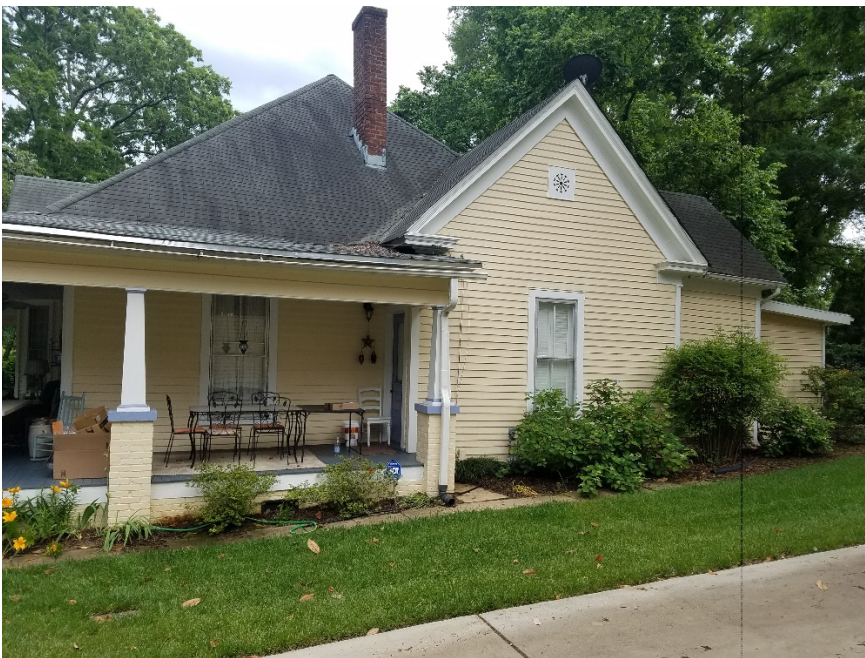
Existing Right (viewed from front) gable. Vent to be replaced with 36"x36" casement window.
